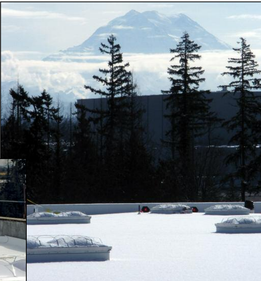
THE WHIRLPOOL DISTRIBUTION FACILITY IN FREDRICKSON WASH. BELOW, A WORKER USES THE ACCUSEAM TOOL.
